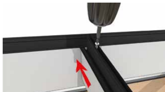
14 Re-tighten the screw in the top of the transom rafter which will pull the joint together and secure.
